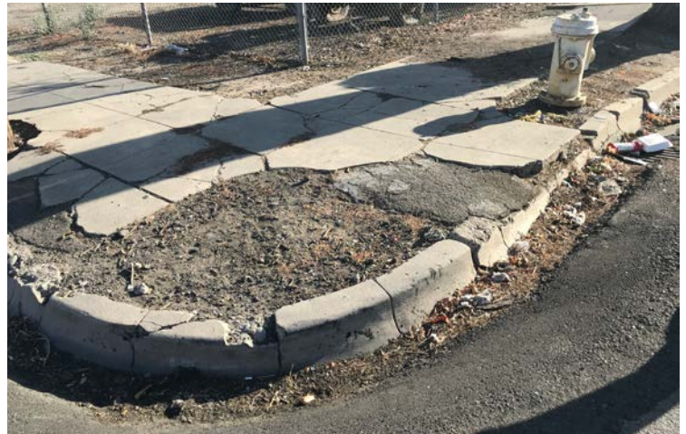
Example of poor maintenance and lack of curb ramps in neighborhood.
