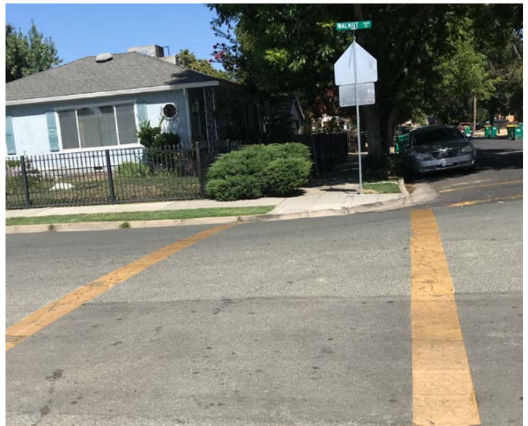
Lack of curb ramps throughout neighborhood.
