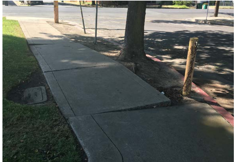
Uplifted sidewalk in front of school..
