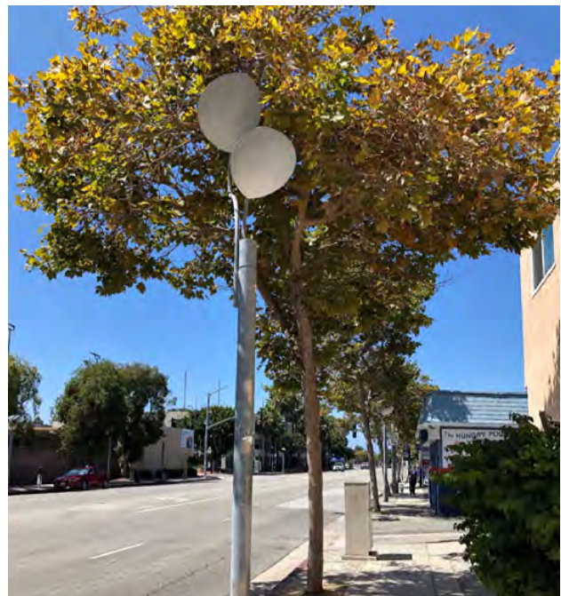
Tree branches block the pedestrian-scale lighting fixture.
