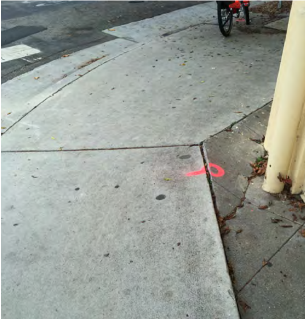
Left: Tree roots uplift the sidewalk at Pico Boulevard/22nd Street.
