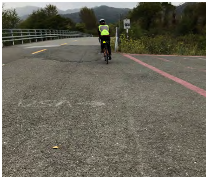
Cracked roadway on Hatchery Road.
