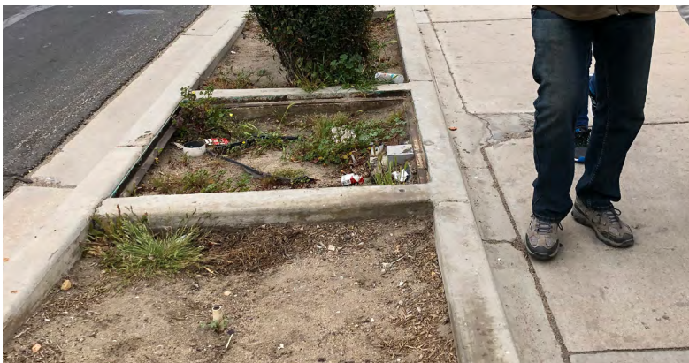
An empty landscaping buffer on 7th Street, just southwest of D Street.
