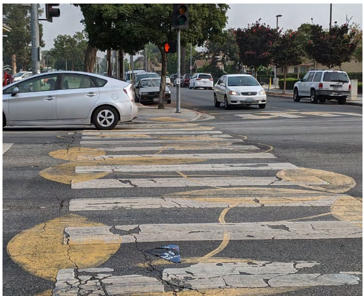
The faded creative crosswalk at the Anaheim Street/Gundry Avenue intersection.
