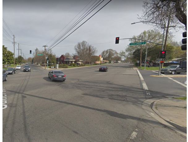
The five crosswalks at the Paradise Avenue/Tuolumne Boulevard intersection are faded and create potential conflict points between pedestrians in the crosswalk and drivers encroaching in the crosswalk.
