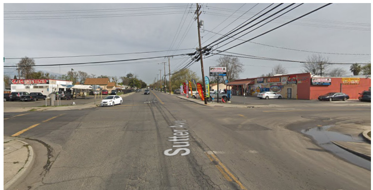
Drivers don't stop ahead of the faded crosswalk markings at the Sutter Avenue/Rouse Avenue intersection. .
