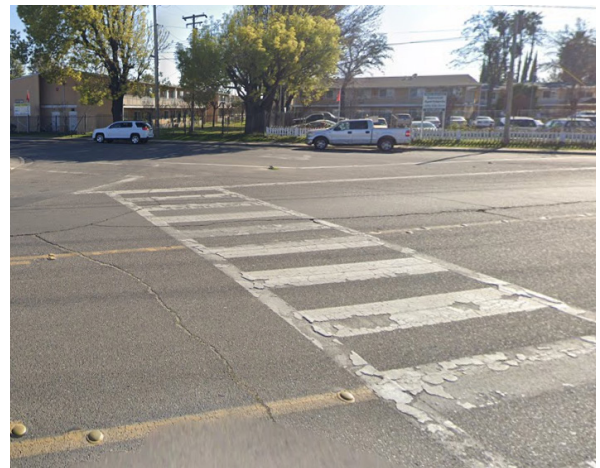
The faded bulb-out marking on the east end of the crosswalk at the Paradise Avenue/Chicago Avenue intersection.
