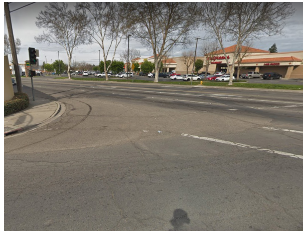
Tire friction marks made by drivers traveling northeast on Paradise Road and turning at a high speed onto Sutter Avenue.
