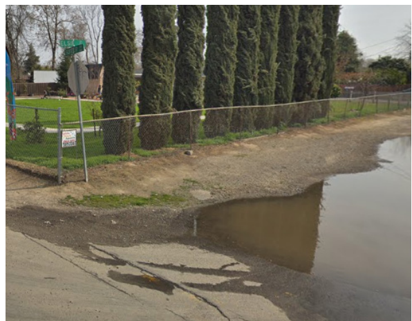
Flooding on Elsie Street forces students to walk in the street because the dirt road gets muddy.
