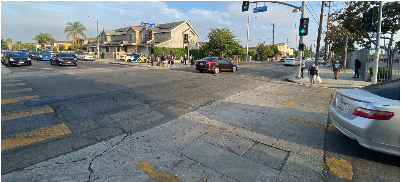
Cracked uneven pavement and faded crosswalk markings at the 67th Street/San Pedro Street intersection
