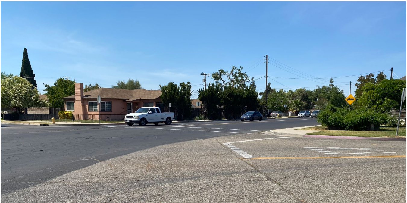
The northern crosswalk of the five-way Lake Street/4th Street/Central Avenue intersection is unmarked and missing curb ramps.
